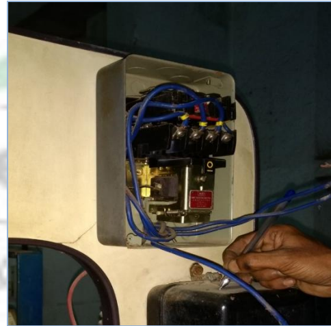
Fig. Obsolete (Not Working) 3 Phase Induction Motor Starter.
